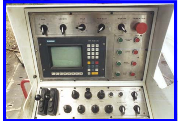
TTM100 operators controls
